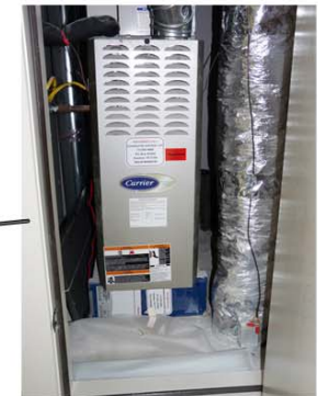
Air handler equipped with outside air damper and electronic control unit ensuring proper outside air exchange rates.
