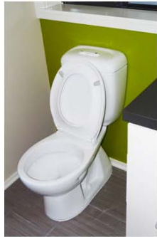
Dual-flush toilet conserves water and bathroom tile contains recycled content.
